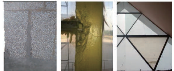
the damaged window with seepage
