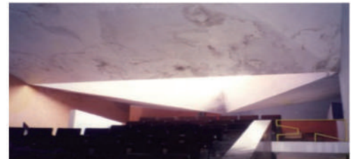
The skylight and seepage condition of the ceiling in auditorium.
