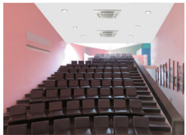
Ceiling A.C. unit in auditorium
