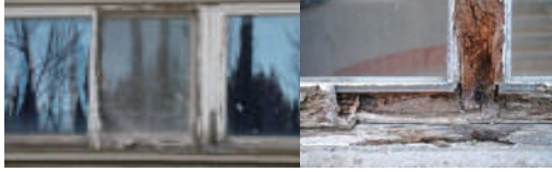
Decay of Windows frames
